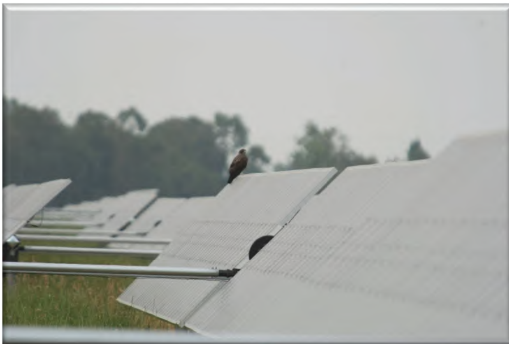
Plate 6. Adult Swainson's hawk perched on solar panel at the McKenzie site. This use of the solar array suggests potential onsite foraging activity.
