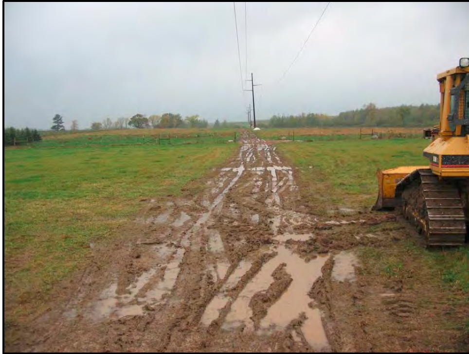
Figure D.2. Minor soil rutting in pastureland.
