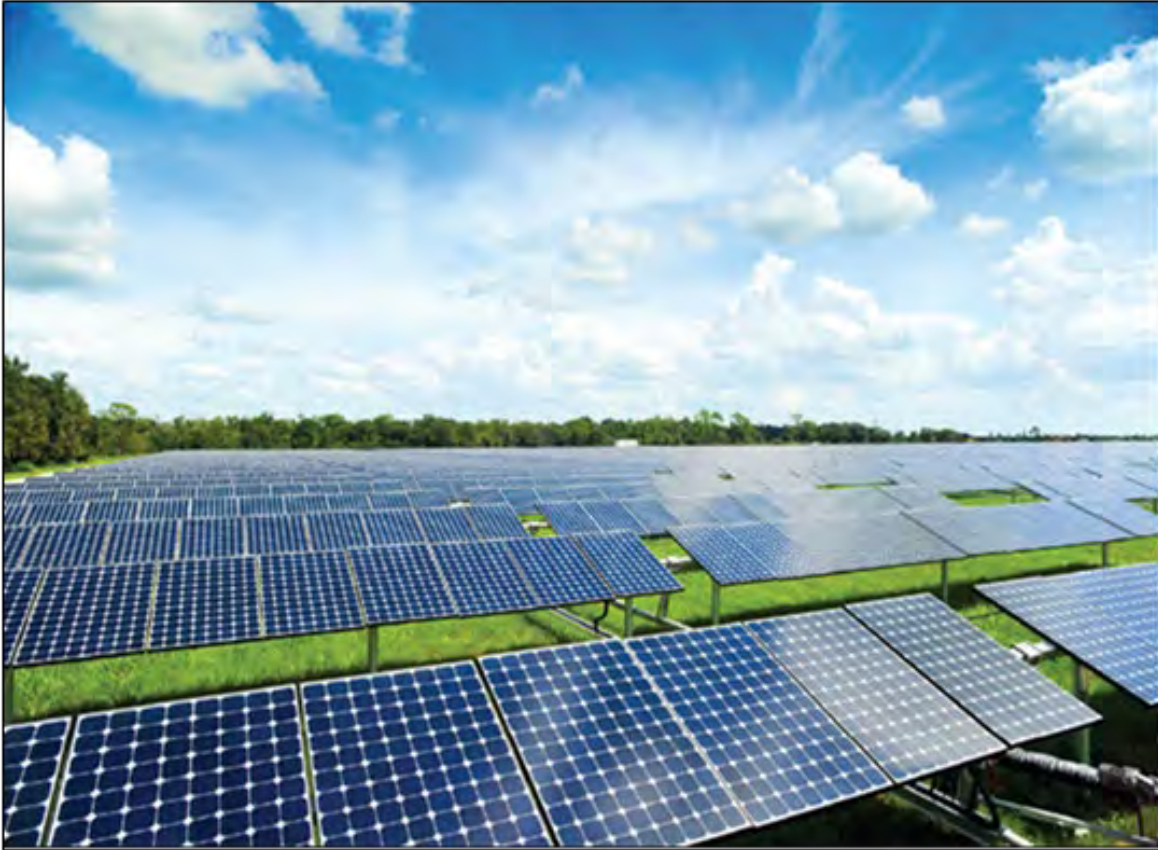
Photo 3.7-5. Single-axis, tracking photovoltaic system with panels close to maximum tilt
