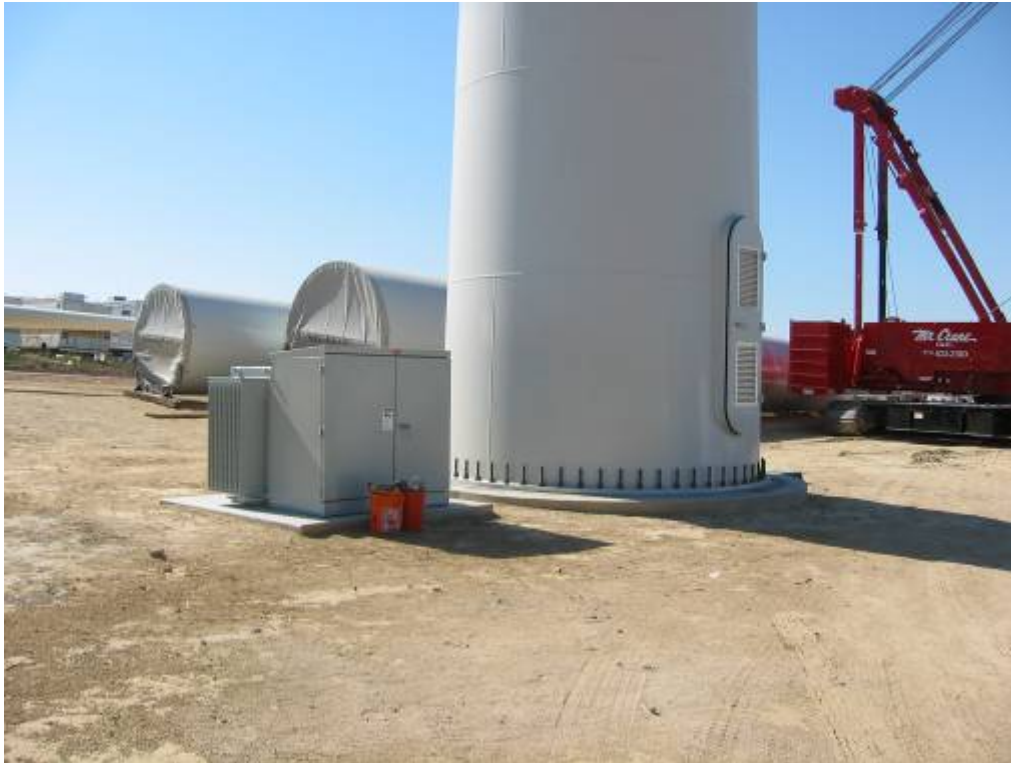
Figure 6-1. Typical Wind Turbine Transformer Arrangement
