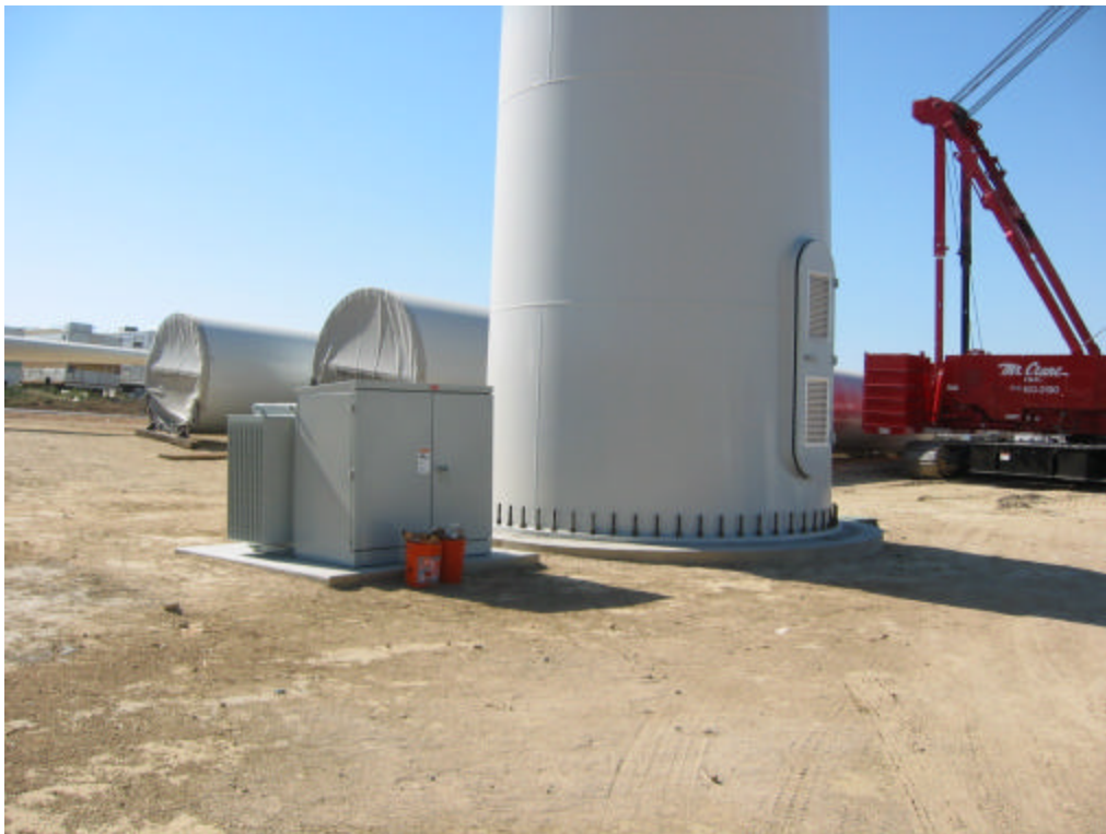
Figure 6-1 Typical Wind Turbine Transformer Arrangement
