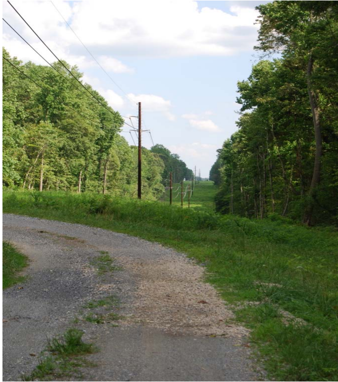
Figure 1-2 Typical View of the Existing 69 kV in Predominately Rural and Forested Areas Source: Black & Veatch
