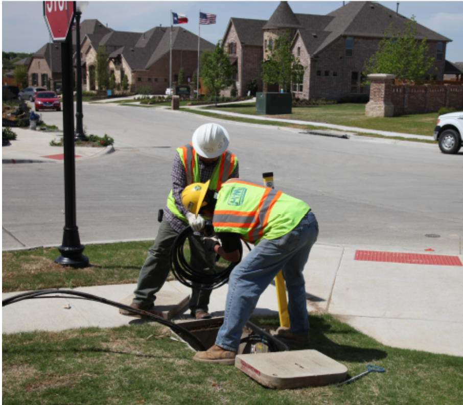
Figure 2-8. A handhole in a suburban neighborhood. Source: Power and Communication Contractors Association
