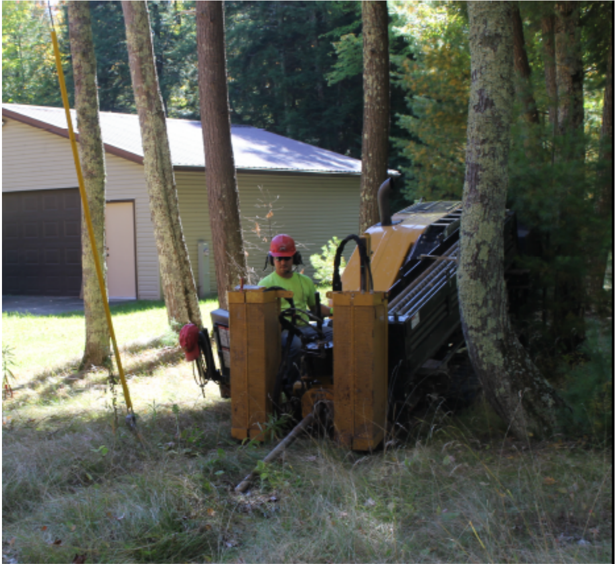
Figure 2-7. Directional Boring in a sensitive area. Source: Power and Communication Contractors Association
