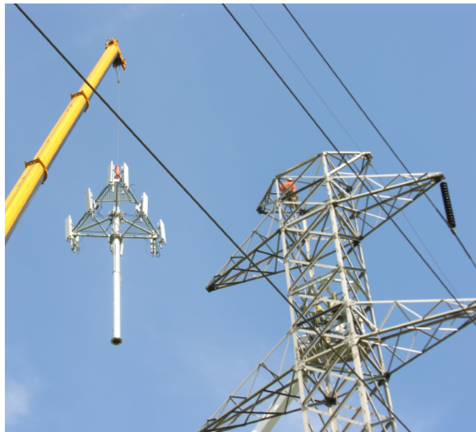
Figure 2-13. Collocation of a cell tower on existing electric transmission infrastructure. Source: Power and Communication Contractors Association
