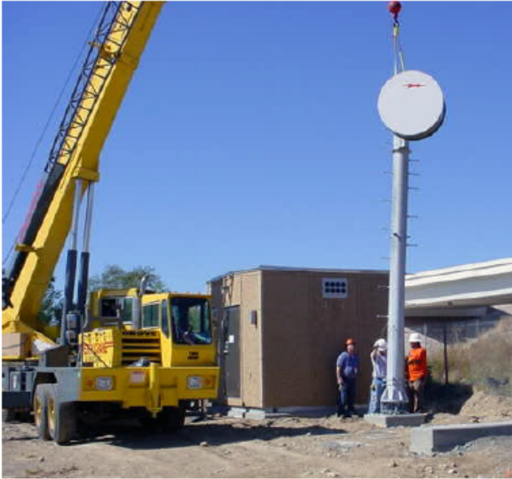
Figure 2-12. Final construction of a microwave tower. Source: Power and Communication Contractors Association
