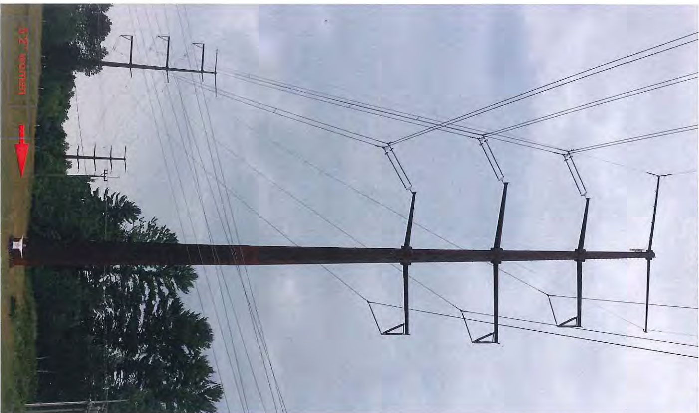
ATC 345,000 volt transmission line, Douglas County, WI
